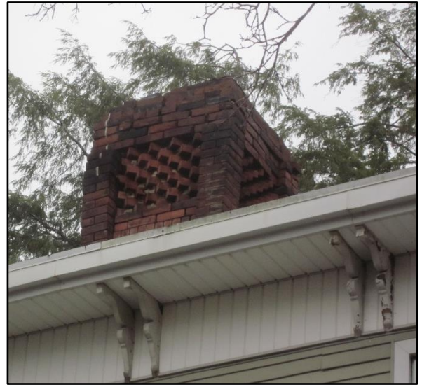
Figure 7. The chimney struck by lightning. Photo by Cynthia Turk, 2023.
